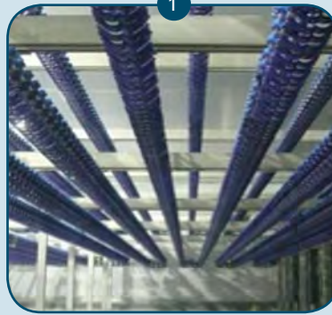
1 New air chiller.
